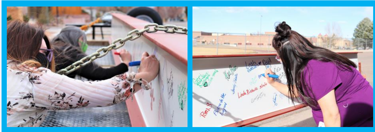
Staff at Pueblo Community Health Center signing a beam in the East-Side Expansion project.
